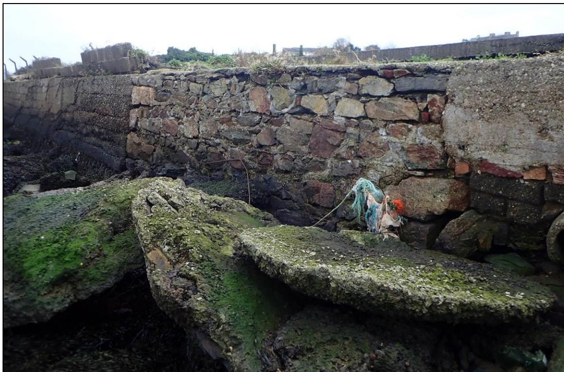
Plate 4: View looking west at river-frontage of Trinity Wharf. The stonework relates to former elements of the dockyard while the later concrete additions either side may mark where infill of the patent and related slipways has taken place.
