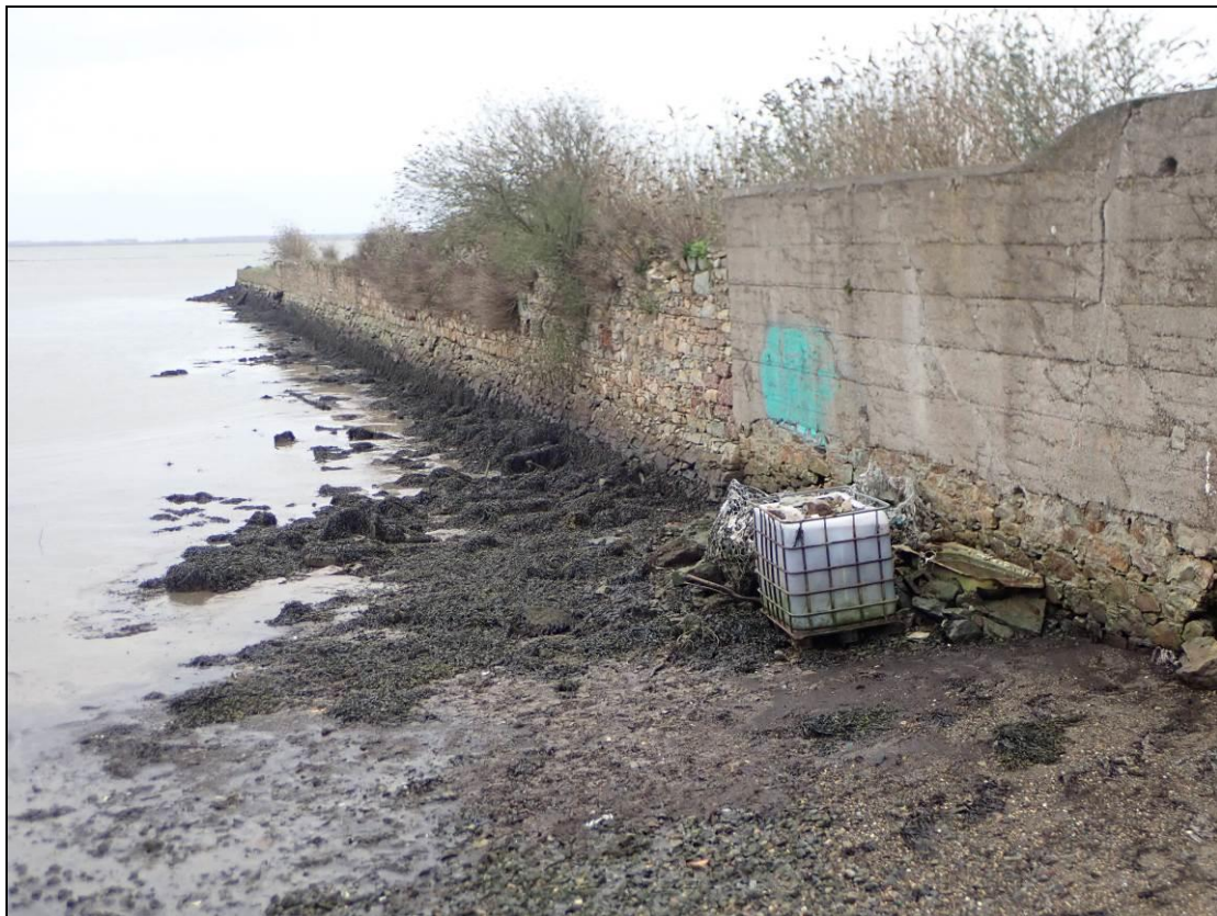
Plate 2: North-facing boundary wall of Trinity Wharf, that served originally to define the edge of the nineteenth-century dockyard. The concrete additions are later.
