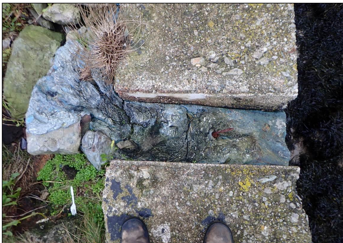
Figure 7: View of molten material that has flowed between concrete copings on the east edge of Trinity Wharf, indicating the intensity of the ironworks activity.
